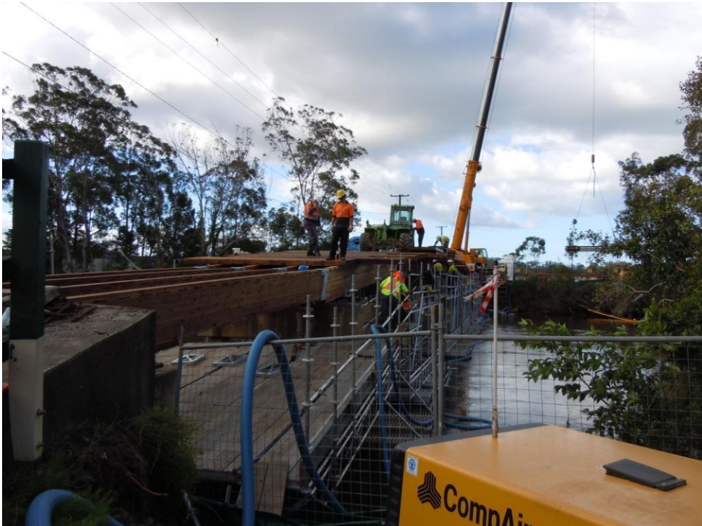
New Penta treated glulam deck panels are laid over the recently installed girders.
