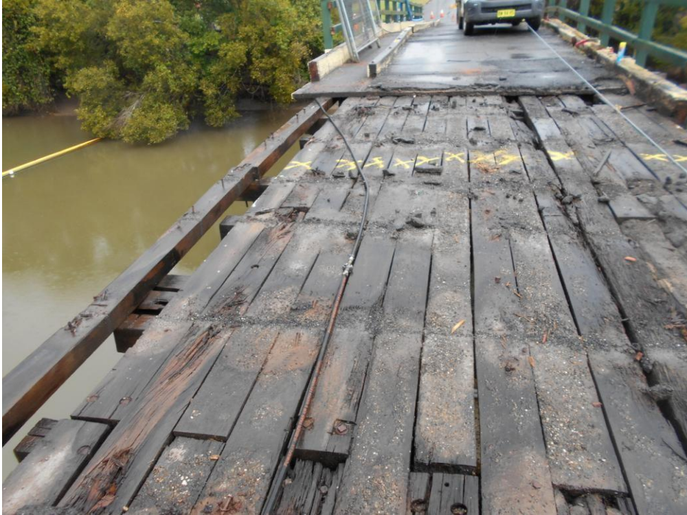
Once the asphalt was removed, the full extent of the deterioration of the deck system was evident.
