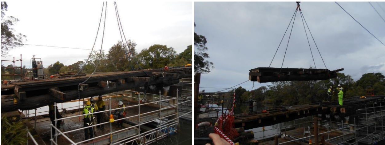
TRS technicians then cut the deck system, girders, and corbels into pieces, which were then removed via crane.
