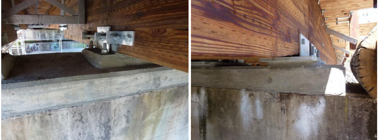
The area between the bottom of the jack-post and the top of the cap is filled with concrete for added strength.
