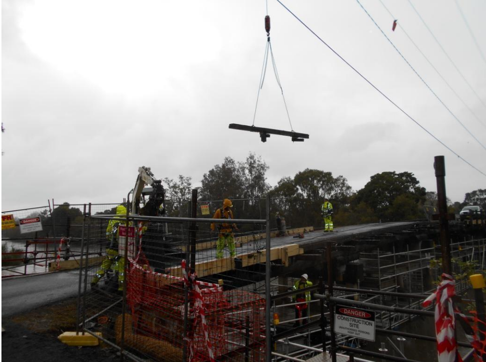
The crane was then used to remove the kerbs from the deck.
