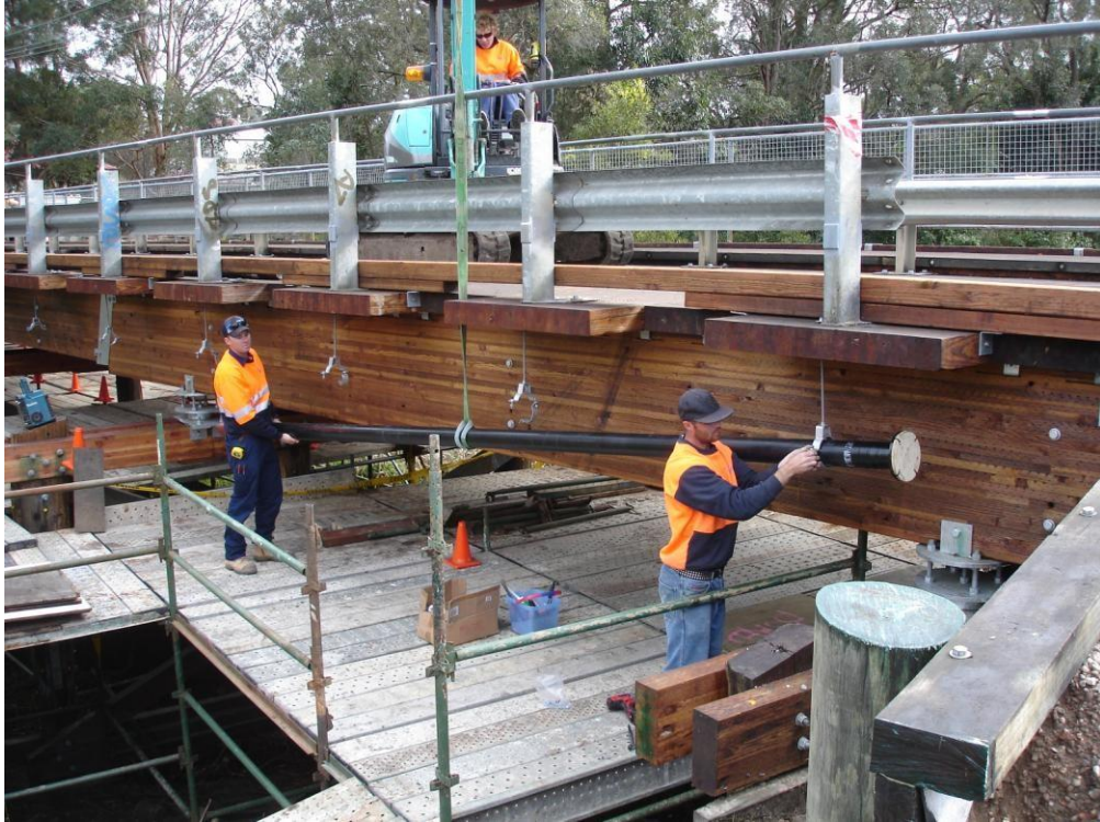
Technicians install a new utility pipe to the exterior of the structure.
