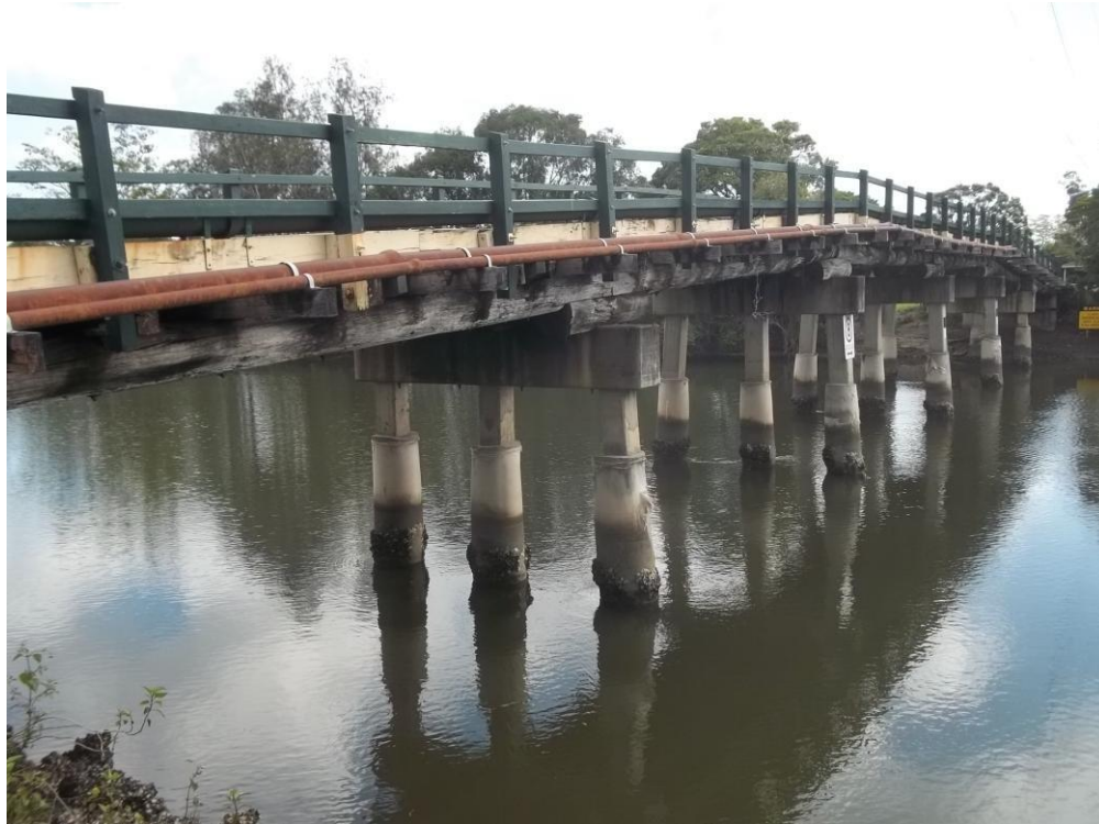
Utility pipes are connected to the side of the bridge.
