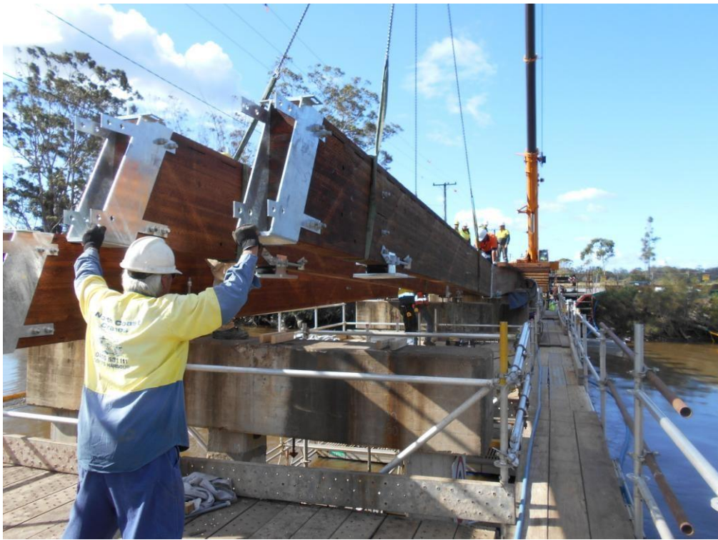
TRS technicians the utilized the crane to install the remaining glulam girders.
