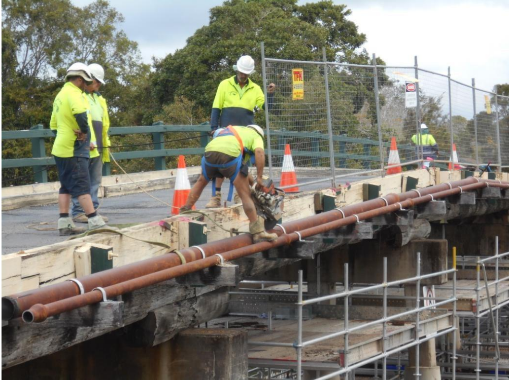
TRS technicians then removed the guardrails, and then cut and removed the utility pipe from the side of the bridge.
