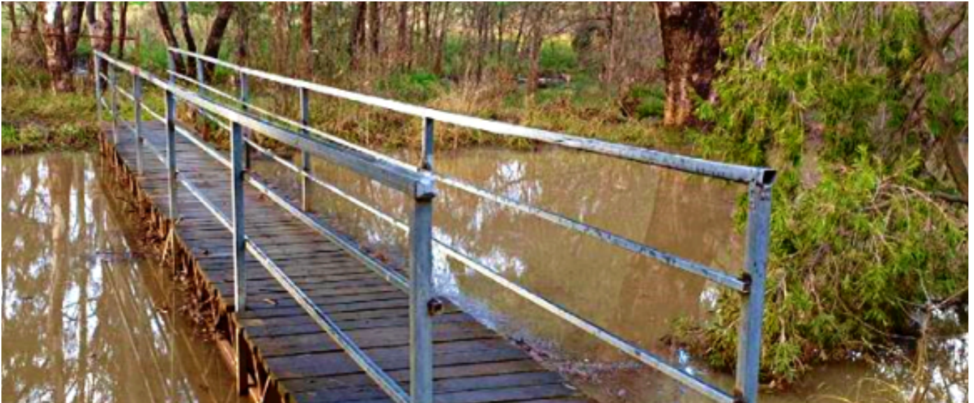
The original Flowerdale lagoon bridge to be replaced as a part of council project.
