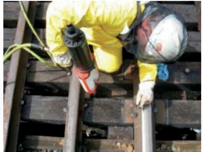
Injecting Structurfill® Epoxy into the chord piles from the top of the bridge
