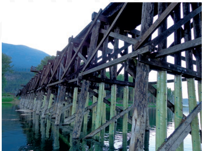
Photo above and to the right shows Retromatrix® High strength fiber wrap on CPR Kootenay Landing Bridge in British Columbia
