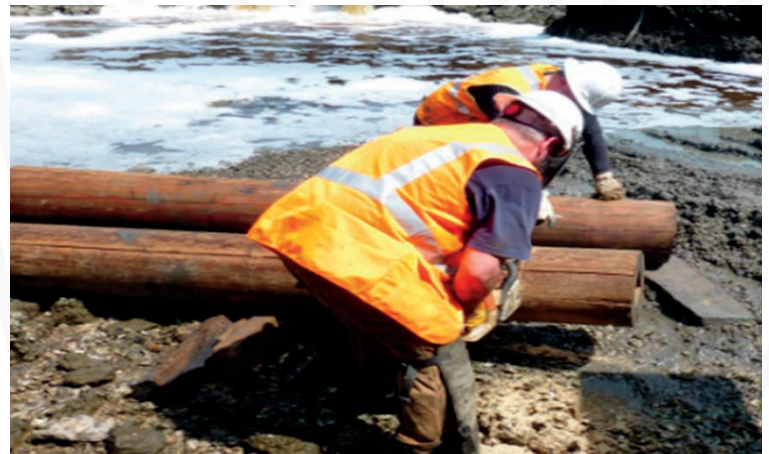
The pre-manufactured DF Pentachlorophenol pressure treated Dutchman's patch is cut to length and ready for installation
